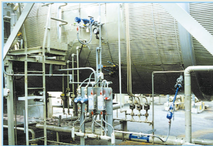
AGAR probes installed on a desalter in the AMOCO Mandan Refinery
