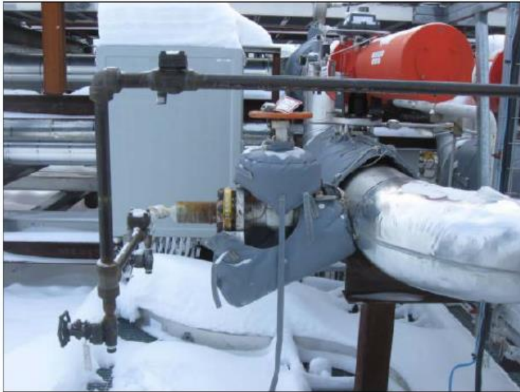
Figure 48: Well R Gas Cross-over Line
